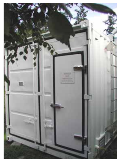
Pilot installatie membraan bio reactor (MBR)
